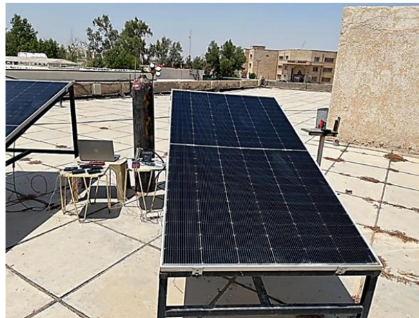
Figure 3 CO 2 gas supply line and distribution system used for rear side cooling of the photovoltaic module.
